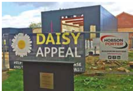
Work in progress at the new Molecular Imaging Research Centre which will open at Castle Hill Hospital next year
