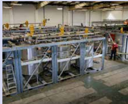
Picture shows the process plant newly installed at HETA's headquarters in Hull.
